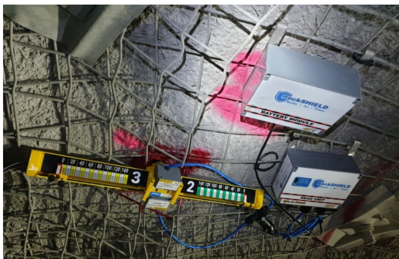
Figure 12 Stage 2 SmartTT and RockSHIELD head unit and battery module at Fosterville Gold Mine
