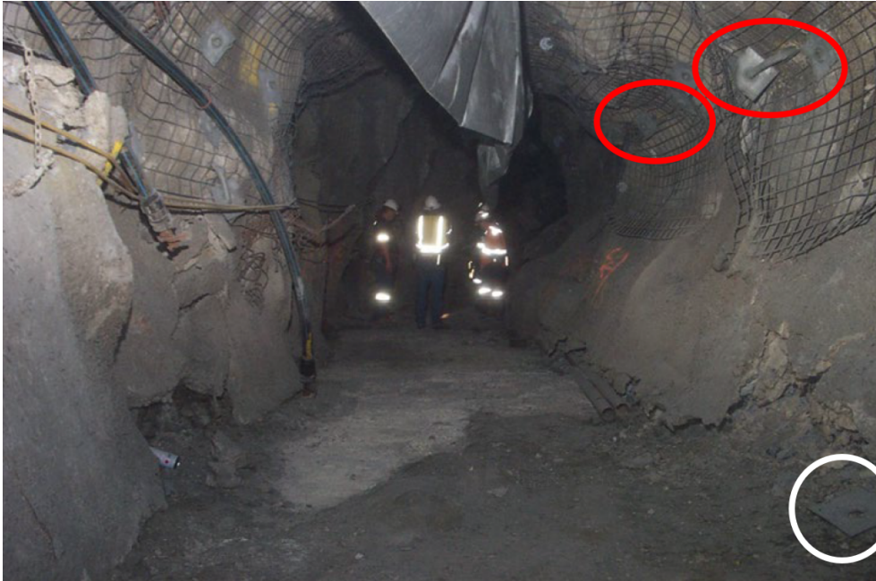
Figure 2 Examples of failed rockbolts due to squeezing ground. Red circles indicate rockbolts that have been pulled out of the wall with their plates still attached but because of their detachment from the wall, they are no longer effective. Note how the plate orientation has been twisted from the original position flush to the wall. The white circle shows a plate that has been detached and has fallen to the ground (ACG 2022)
