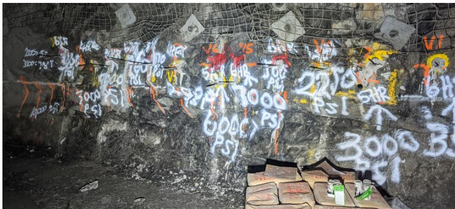
Figure 2 Post pull testing cable bolts with pressures in psi recorded on the wall
