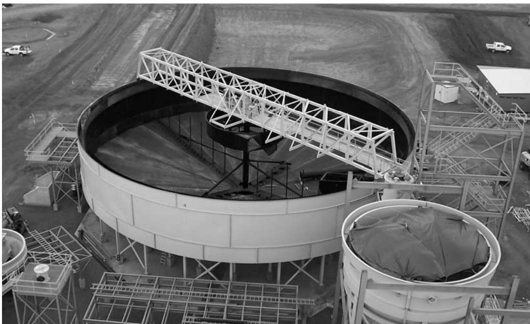
Figure 4 Example of 33 m thickener installation completed by six men in three weeks
