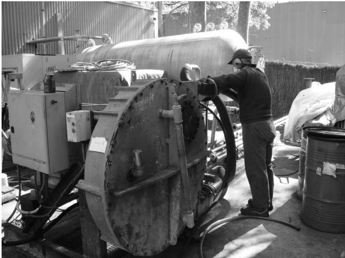
Figure 7 Breidel SPX100 hose pump
