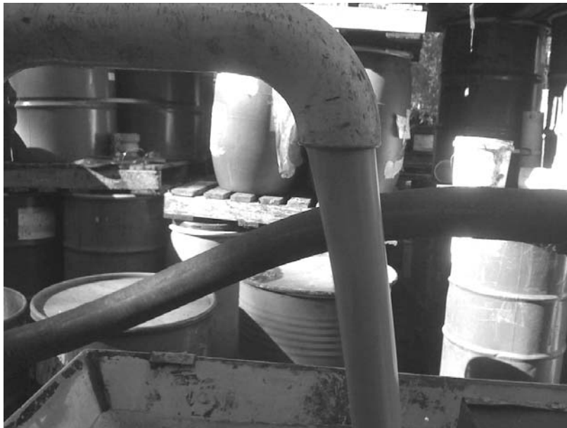
Figure 9 Slurry discharge from pilot plant pipeline
