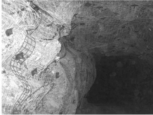
Figure 2 Squeezing in haulage drift at LaRonde Mine
