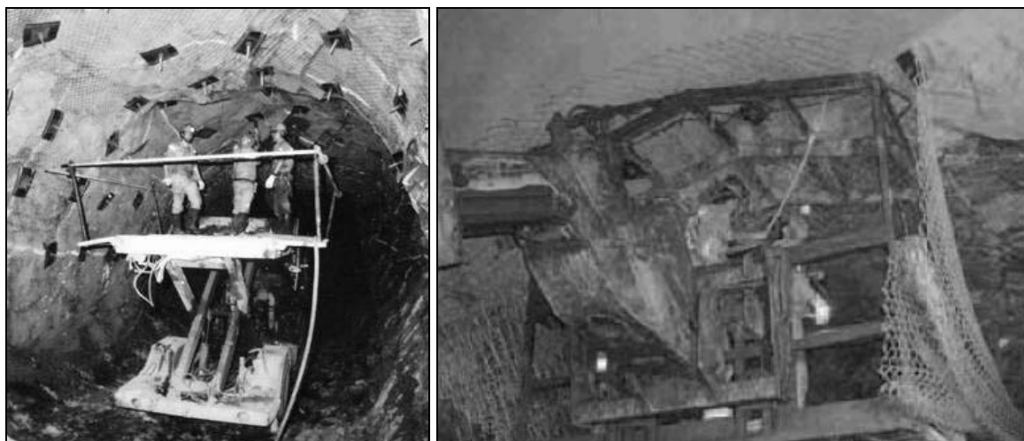
Figure 9 Manual installation of chain-link mesh with scissor lift and installation basket on tool carrier
