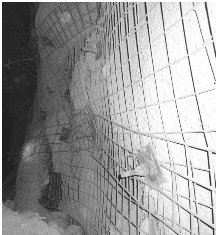
Figure 2 Large wall bulking contained by yielding support
