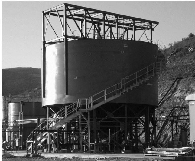
Figure 1 Typical deep cone thickener
