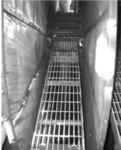
Figure 7 Walkways between the filter discs permit easy and safe access to segments for quick re-clothing
