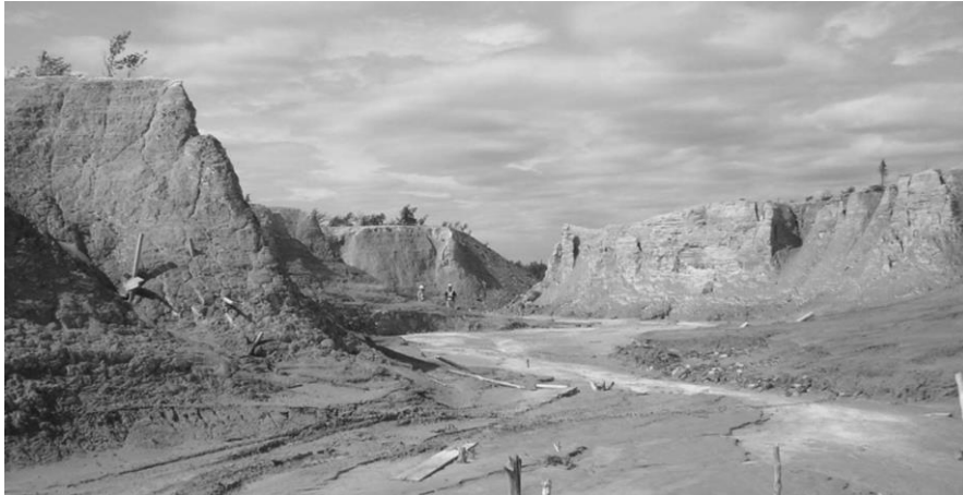
Figure 4 Internal dam breach at Coniaurum tailings facility
