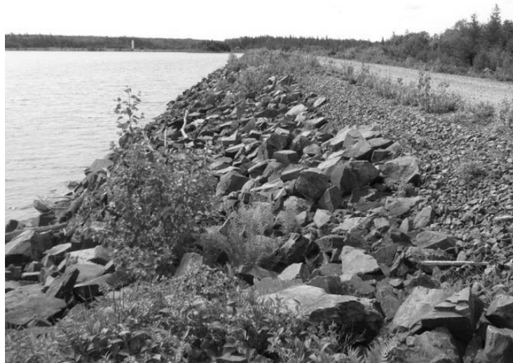
Figure 8 Typical upstream erosion protection for a tailings facility with a water cover
