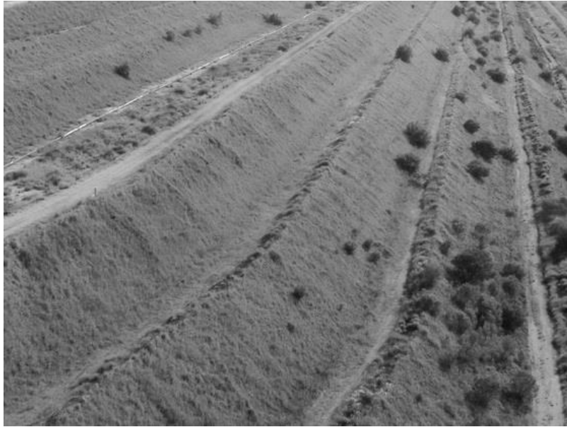
Figure 3 View of the step-in and capping for protection on the sides of the platinum tailings dam
