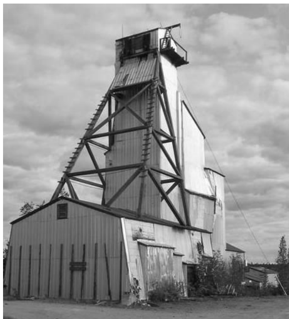
Figure 2 Former discovery mine headframe, Northwest Territories, Canada (photo courtesy Aboriginal Affairs and Northern Development Canada)
