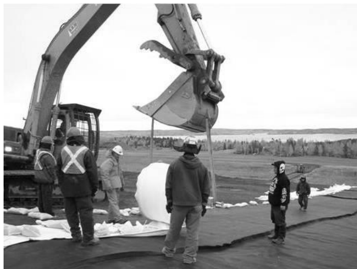
Figure 5 Unrolling geomembrane panel for landfill cover at the former discovery mine, NWT (photo courtesy D. Johnson (with permission of Aboriginal Affairs and Northern Development Canada))
