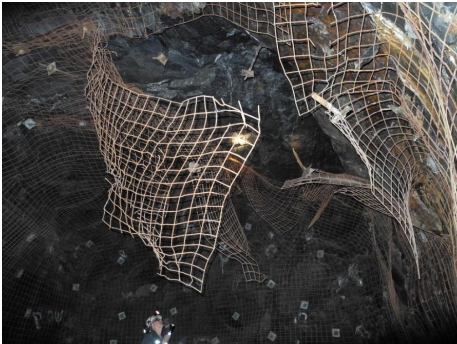
Figure 2 Approximately 4 tonnes of material were displaced at the back of the 7400 powder magazine on 18 May 2011, following CR1418 rockburst
