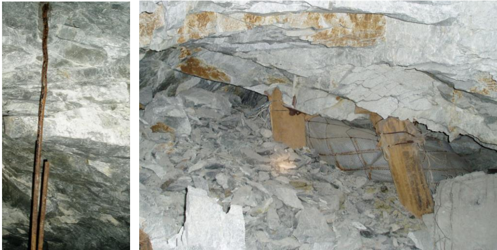
Figure 4 Observations of damage (left) naked tendons (right) punching of props
