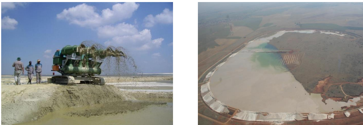
Figure 4 Cyclone TSF built with tracked cyclone units
