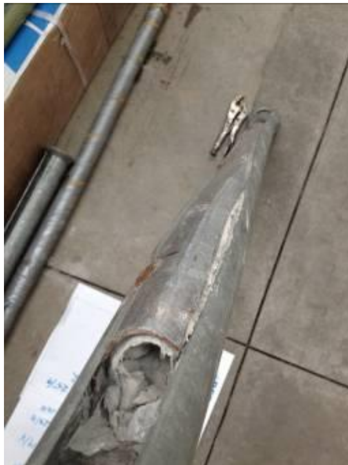
Figure 5 Beginning of Stiff Set bolt flap rupture
