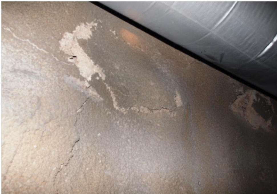
Figure 2 Unstable slabs of fibrecrete
