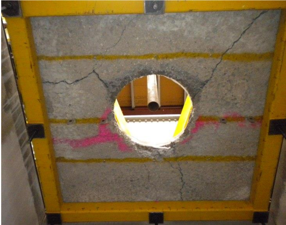
Figure 12 Cracking and punch through failure for sample 4
