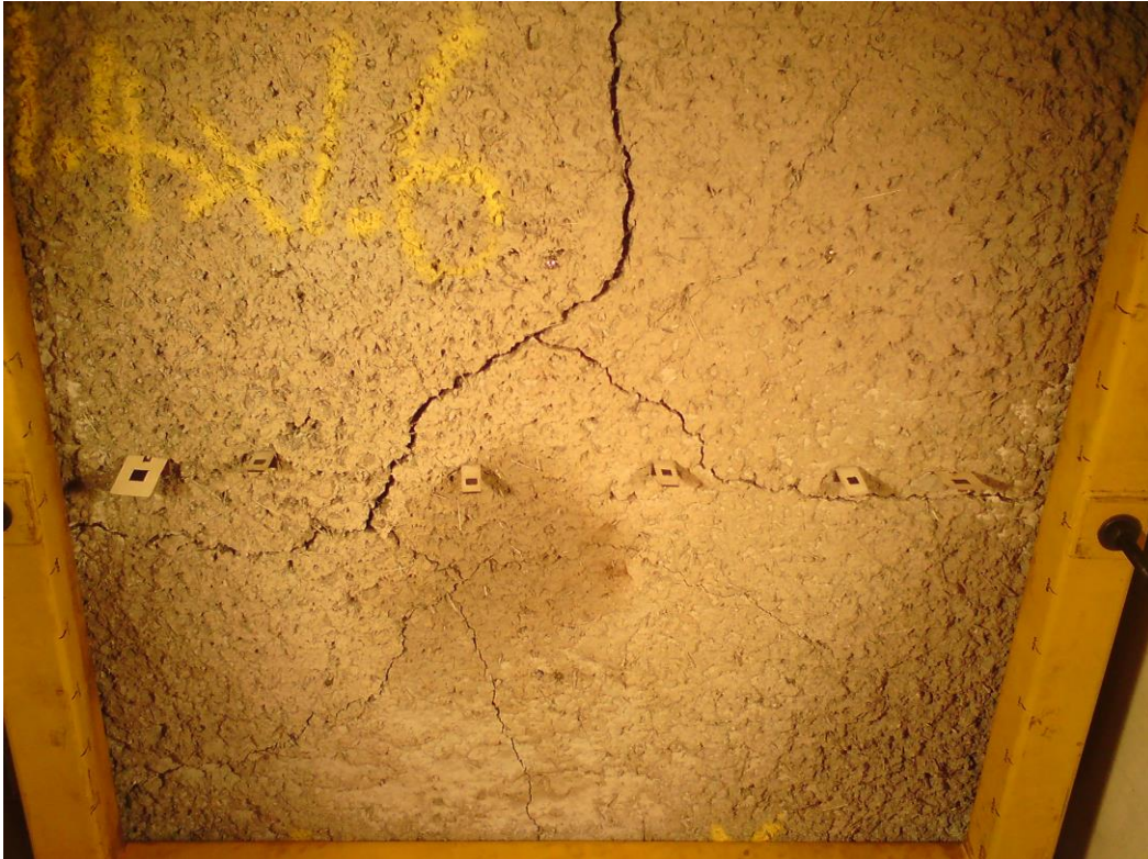
Figure 8 Crack pattern after second test on sample 1
