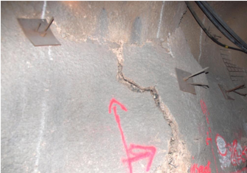
Figure 4 Shotcrete failure due to movement at an excavation wall
