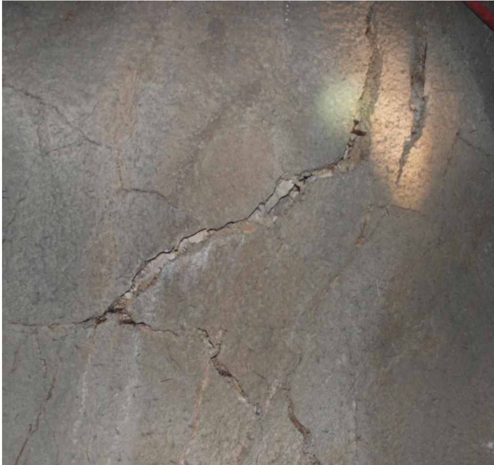
Figure 3 Shotcrete tensile crack opening exceeding the fibre length
