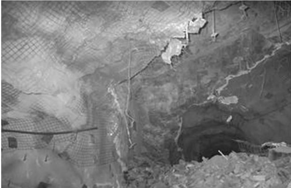
Figure 4 Photograph of a localised incidence of seismically induced damage. It is noted that the surrounding support to the damage area is showing no signs of loading
