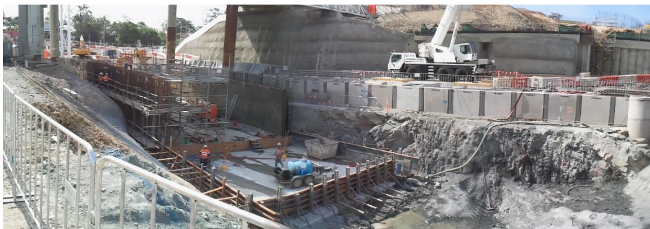
Figure 6 Completed anchored soil nail abutment wall (background) with the ventilation tunnel and drainage structure in the foreground
