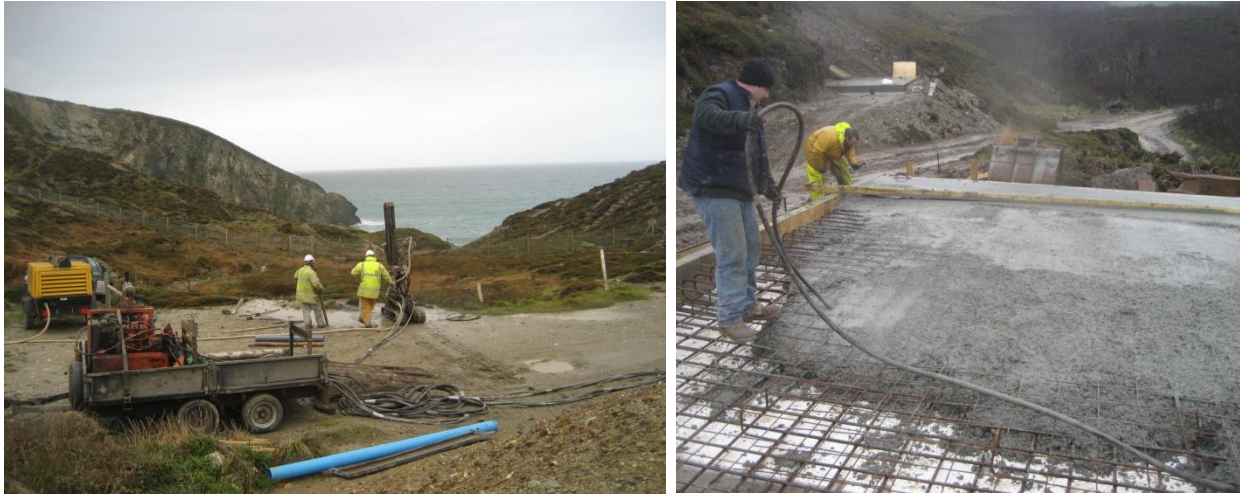
Figure 12 (a) Drilling into the adit to allow water sampling; and (b) shaft capping at Dump D – the cap at Ladderway Shaft is in the background
