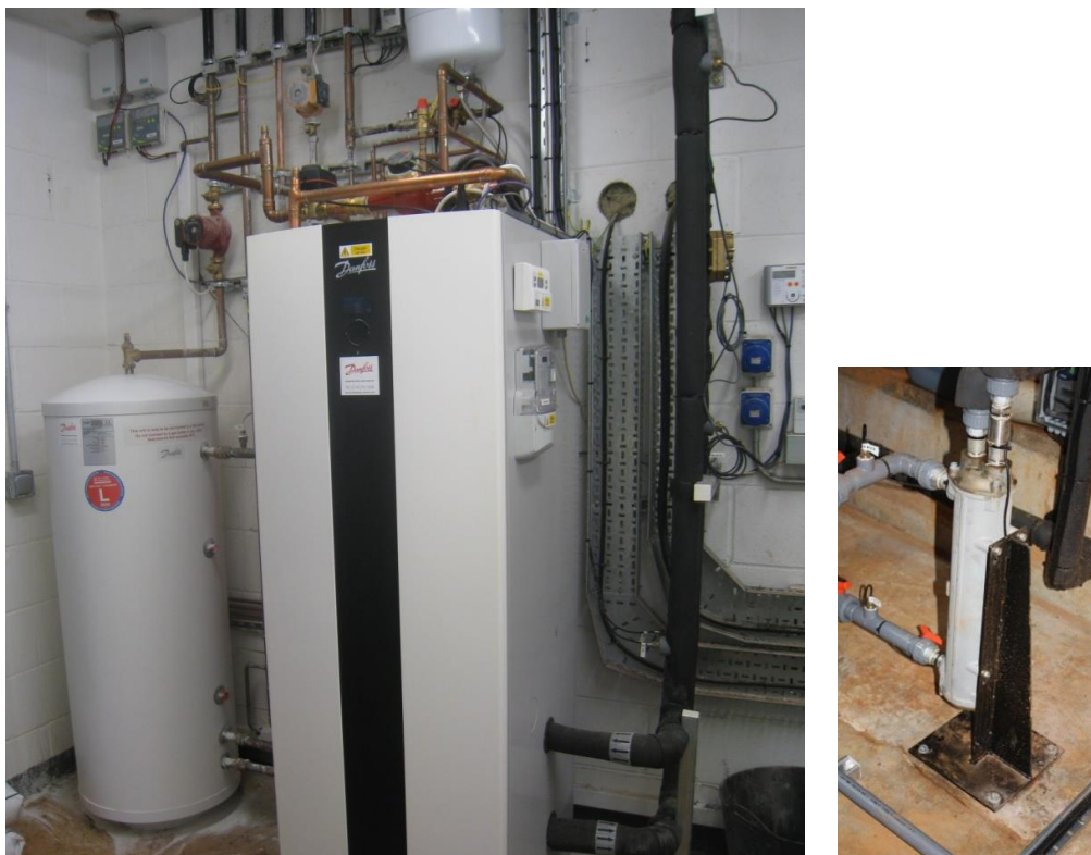
Figure 2 Heat pump (centre) and buffer tank (left) within chemical store room; inset shows tube in shell heat exchanger, which is coupled to the mine water feed
