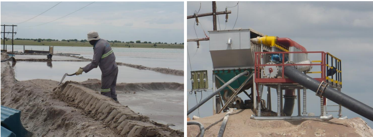
Figure 5 Cyclone pumping into paddock
