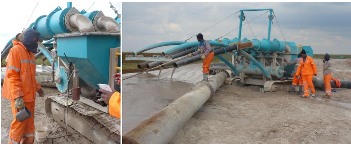
Figure 3 Site test unit
