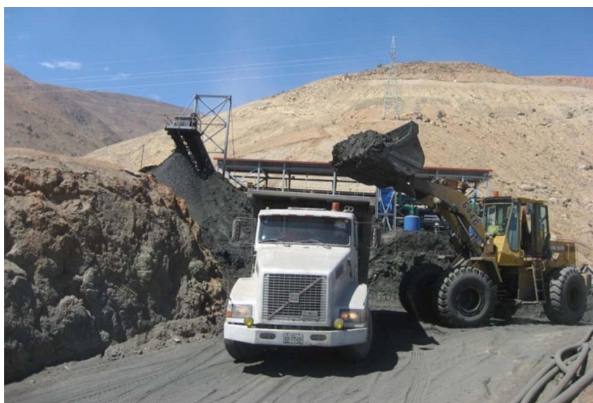
Figure 10 Transportation – FT disposal by trucks (Cerro Lindo Project)
