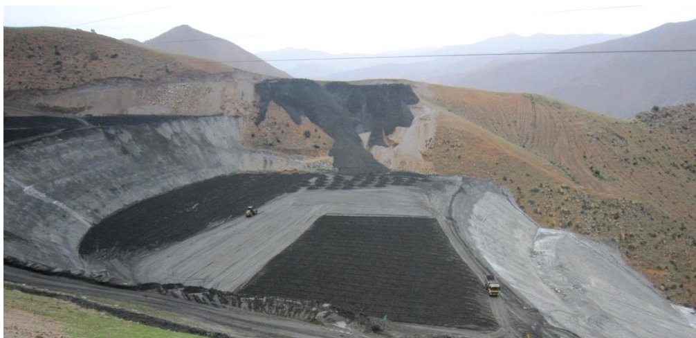
Figure 12 Views of the discharge and drying operation of tailings (Cerro Lindo Project)
