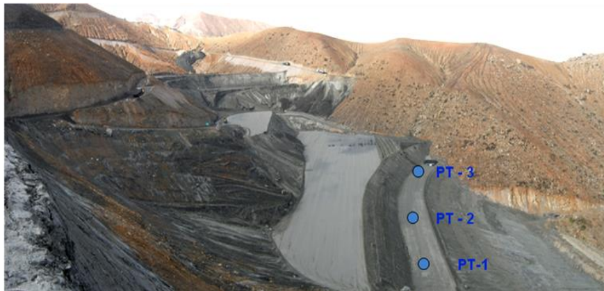
Figure 14 View of the installation points of Casagrande type piezometers, SPT tests and moisture in depth
