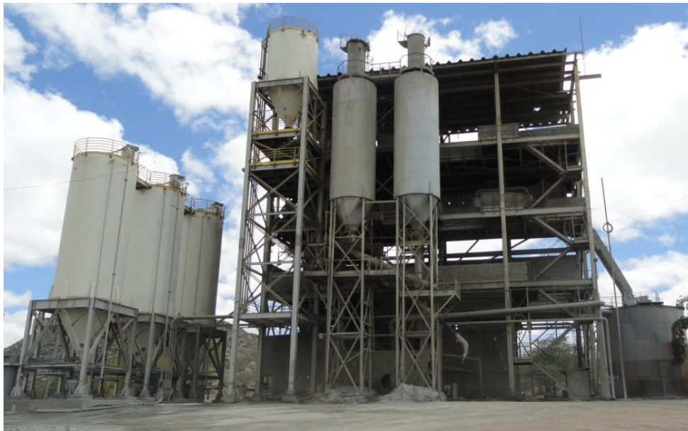
Figure 10 Paste fill plant
