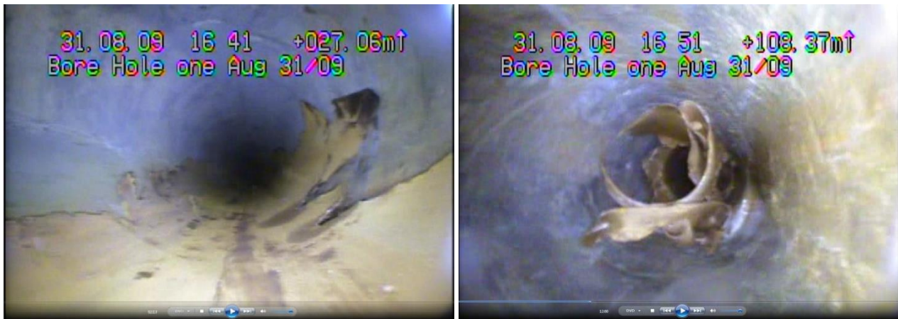
Figure 1 Borehole wear beyond casing into host rock (left) and peeled casing resulting in blockage (right)
