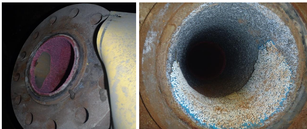
Figure 3 Increased ceramic wear localised at transition from loop to borehole (left) and patch of similar wear after 1.5 Mt of paste fill service (right)
