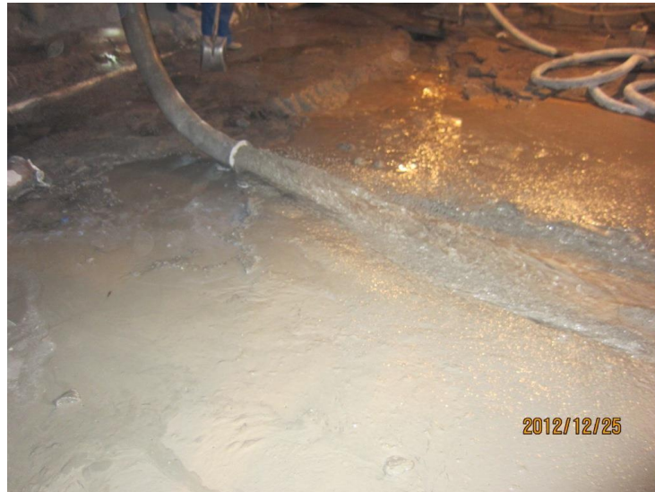
Figure 2 Slurry discharged from the bottom of a large mixer
