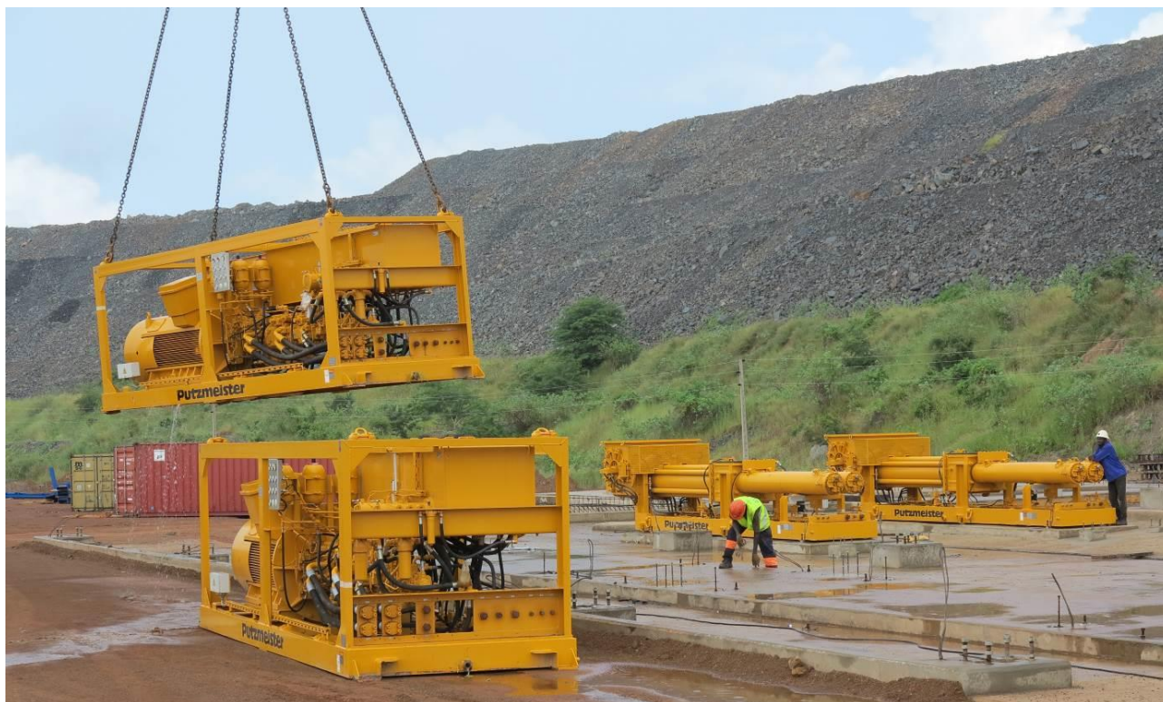
Figure 6 Paste pumps positioning
