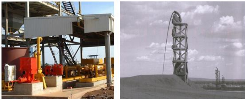
Figure 11 Pumping plant (left); and distribution tower at disposal site (right)
