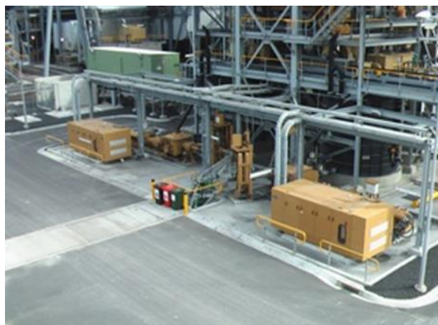
Figure 17 Redundant ash preparation and pumping plant at Kogan Creek
