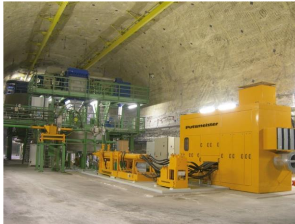
Figure 16 Pumping facility for underground recovery plant in Unterbreizbach
