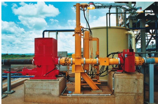
Figure 9 Scraper pig gate; damper; gate valve (left to right)
