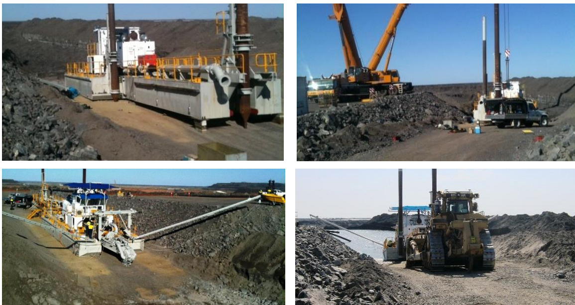
Figure 2 The dredge being assembled on the ramp after mobilisation to site. Once the starter pond had been filled, a dozer was used to push the dredge into it
