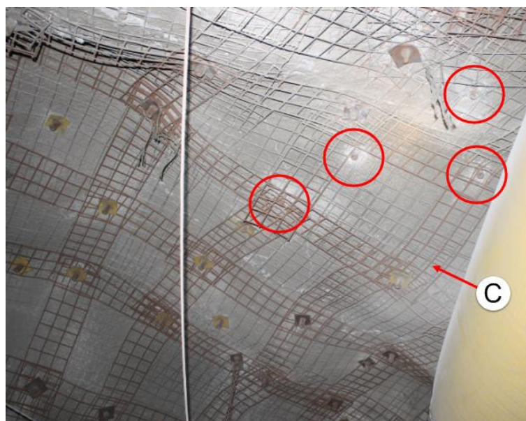
Figure 12 Kidd 2011 rockburst 7000L 01S and S46 intersection roof bulking
