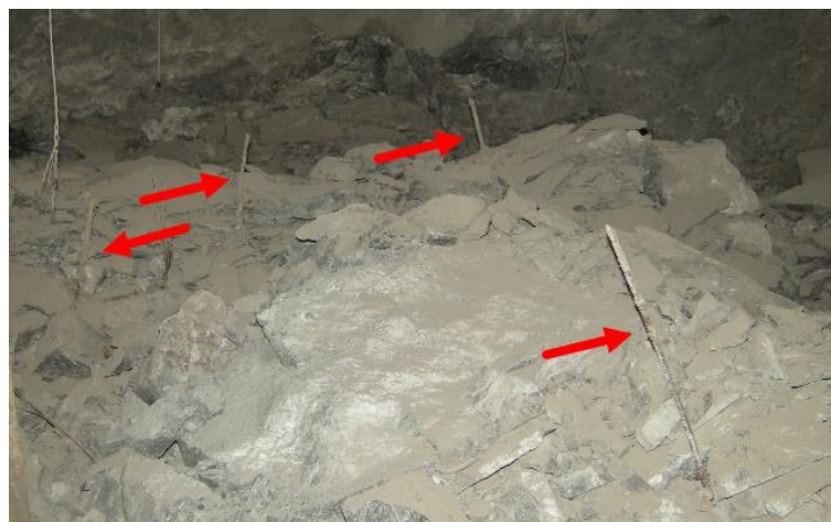
Figure 5 Kidd 2009 rockburst 6800L 74XC intersection with 68-01 Dr. S. Note rebar protruding vertically
