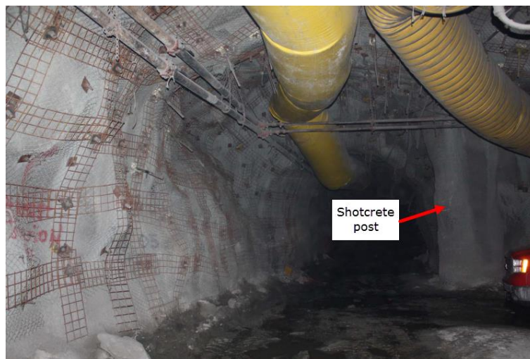
Figure 14 2011 Kidd Mine rockburst 7100L 84XC intersection prior to damage. Photo is looking northwest and 84XC is situated behind the red truck
