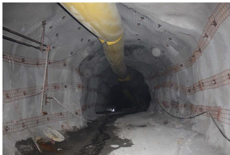
Figure 15 2011 Kidd Mine rockburst 7100L 84XC prior to damage. Photo is looking northeast, at the final repair surfaces put in place after the 2009 event on the same structure
