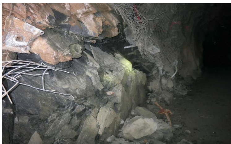
Figure 2 Example of bulking of the lower wall towards the excavation. The buckling action is facilitated by intense foliation surfaces dipping steeply towards the excavation
