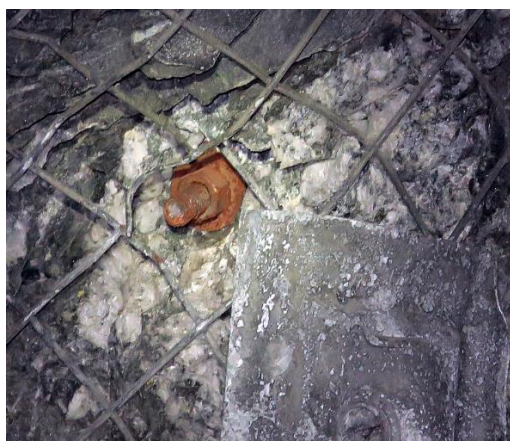
Figure 3 Example of a hybrid bolt that has lost its bearing plate and is being sucked into the rock mass
