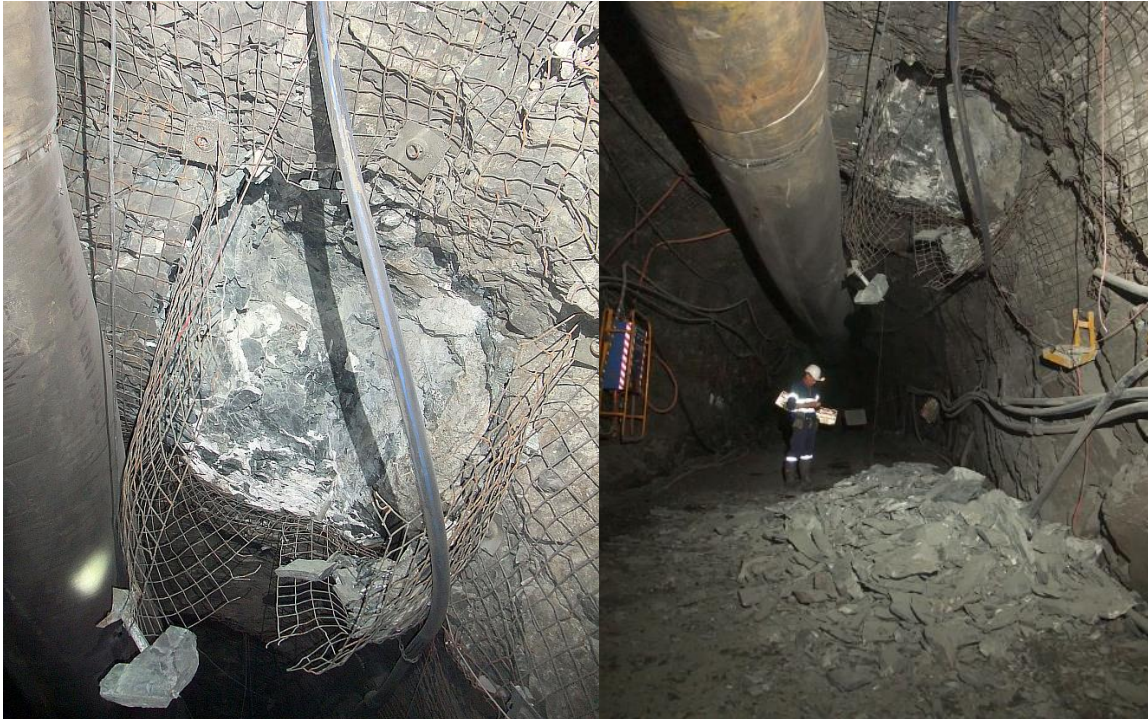
Figure 1 Seismic damage mobilises rock behind the mesh to overload the support scheme (left). Note the two adjacent mesh sheets have parted at the overlap location. Rupture of strands and/or the surface plate fixture occur as the mesh pulls over the plate. This allows release and unravelling of rock from behind the mesh
