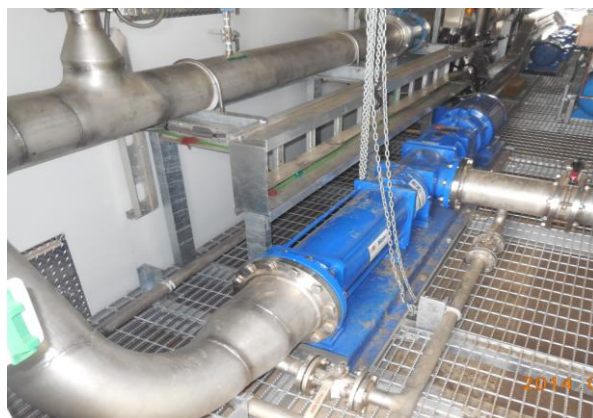
Figure 11 Typical modular plant polymer dosing pump system
