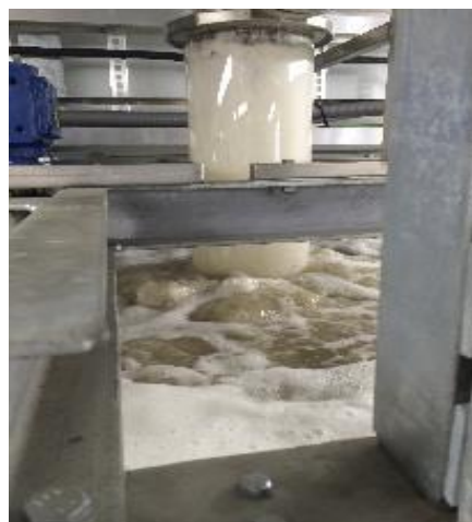
Figure 6 Foam formation due to process water quality
