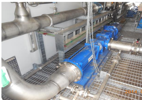
Figure 11 Typical modular plant polymer dosing pump system
