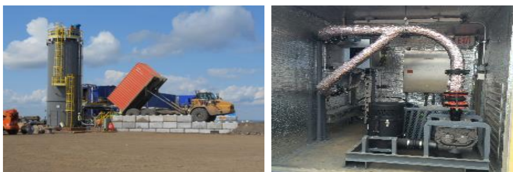
Figure 1 Polymer off-loading facility and equipment
