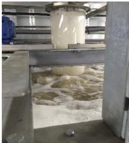
Figure 6 Foam formation due to process water quality
