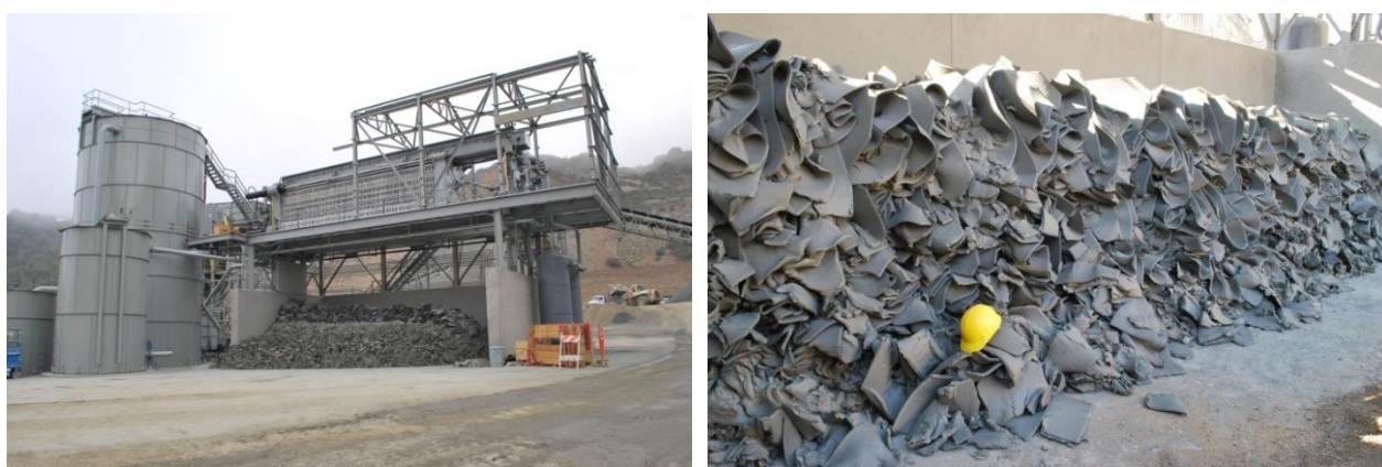
Figure 3 8 m paste thickener and 2 x 2 m recessed plate press (Left) and “Washed Levy Fill” (Right)
