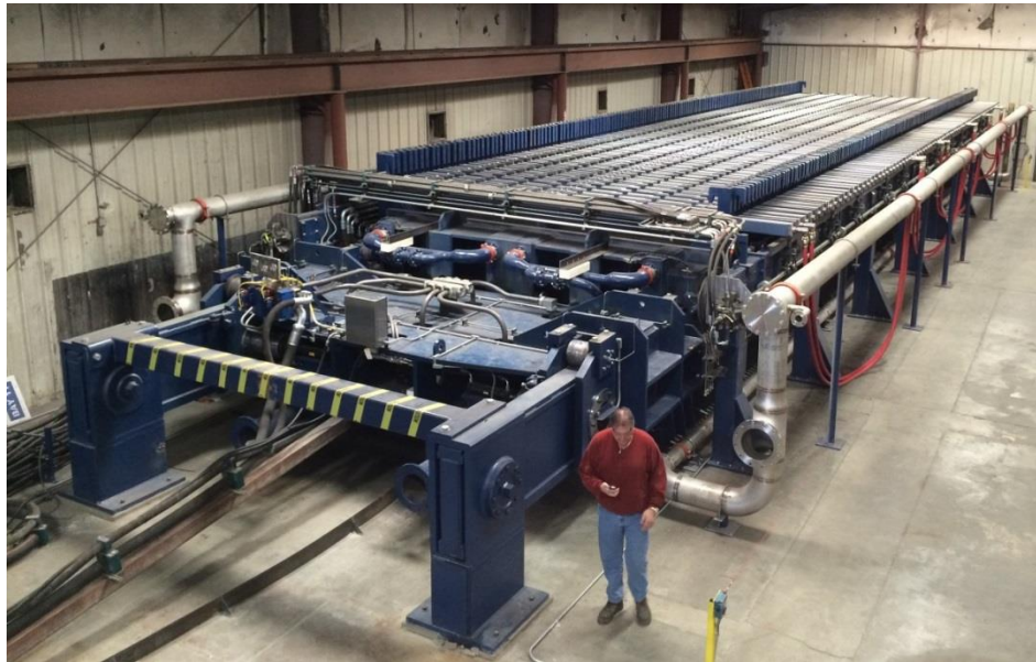
Figure 2 The Colossal filter press at the fabrication facility
