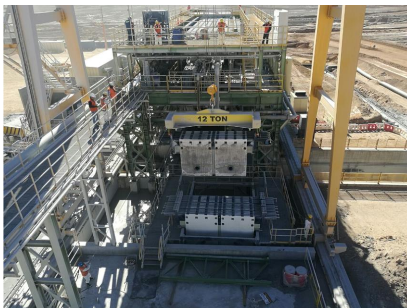
Figure 5 Gantry crane shown lifting filter plates from the maintenance racks to the filter
