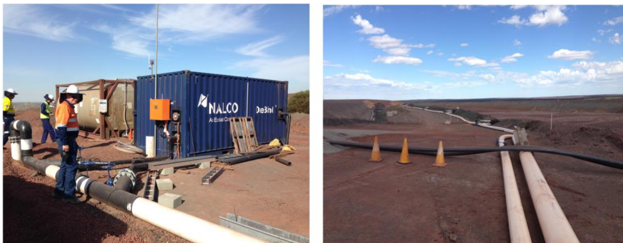
Figure 16 Mobile containerised WaterShed system at Duke TSF
