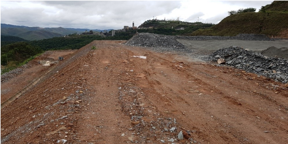
Figure 8 Co-disposal of tailing and waste at the old open pit Cuiabá Mine
