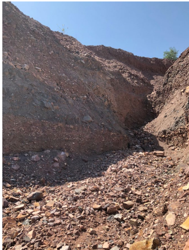
Figure 1 Waste rock dump erosion resulting from inadequate drainage controls
