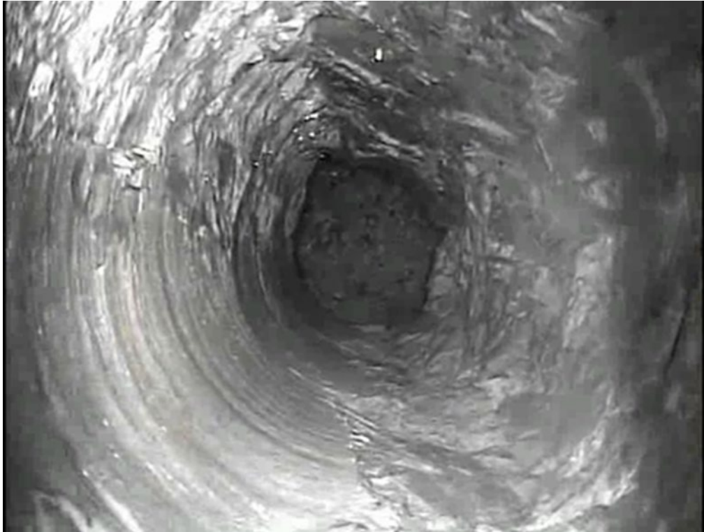
Figure 1 Stability problem after reaming, with difficulty to take down the reaming head and change cutters due to large convergence
