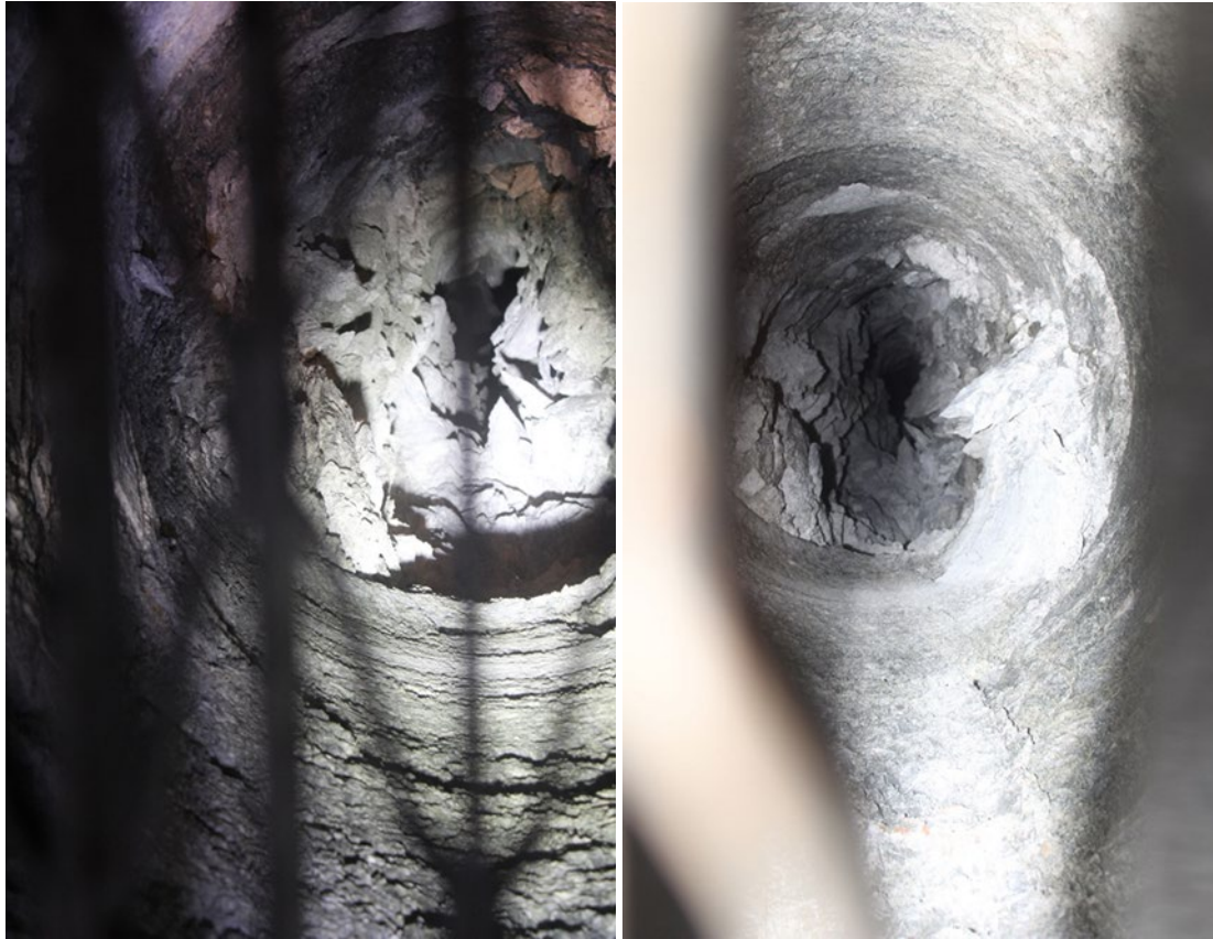
Figure 4 Views down slot raise soon after completion, showing severe crushing and squeezing close of raisebore
