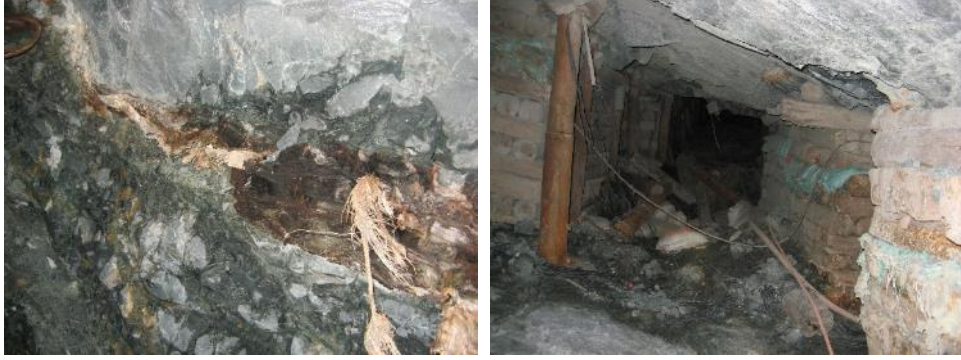
Figure 7. Photographs illustrating the typical mining conditions in the remnants shown above. The photograph on the left illustrates the holing into the old mining area. Total closure occurred as seen by the compressed pack (brown patch in the face). The photograph on the right illustrates the low rate of closure in the remnant in spite of a very high simulated APS value
