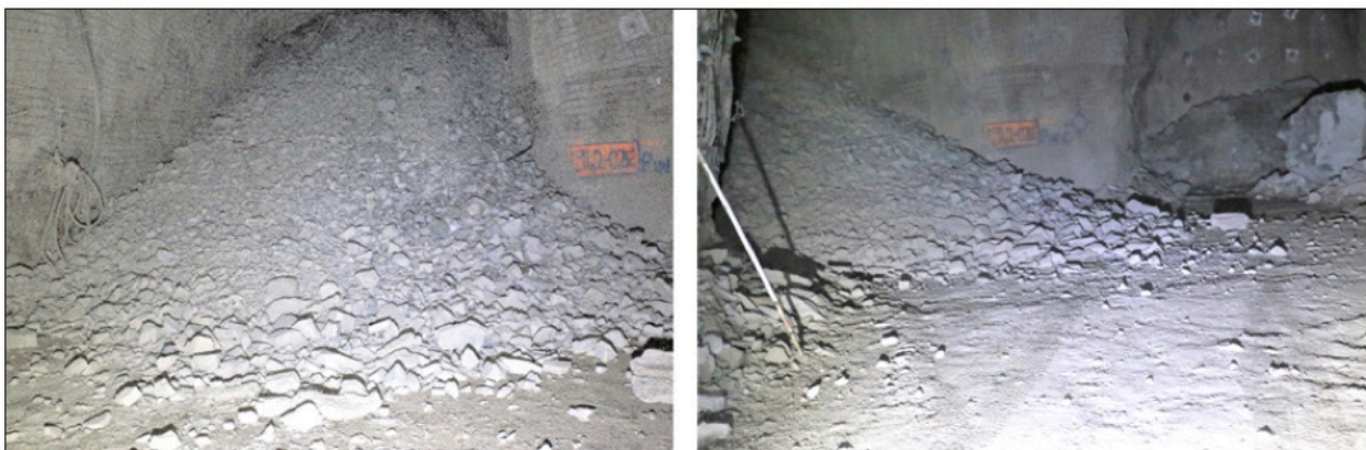
Figure 12 Example of post blast inspection showing blast ejection and fragmentation for 02E Slot shot
