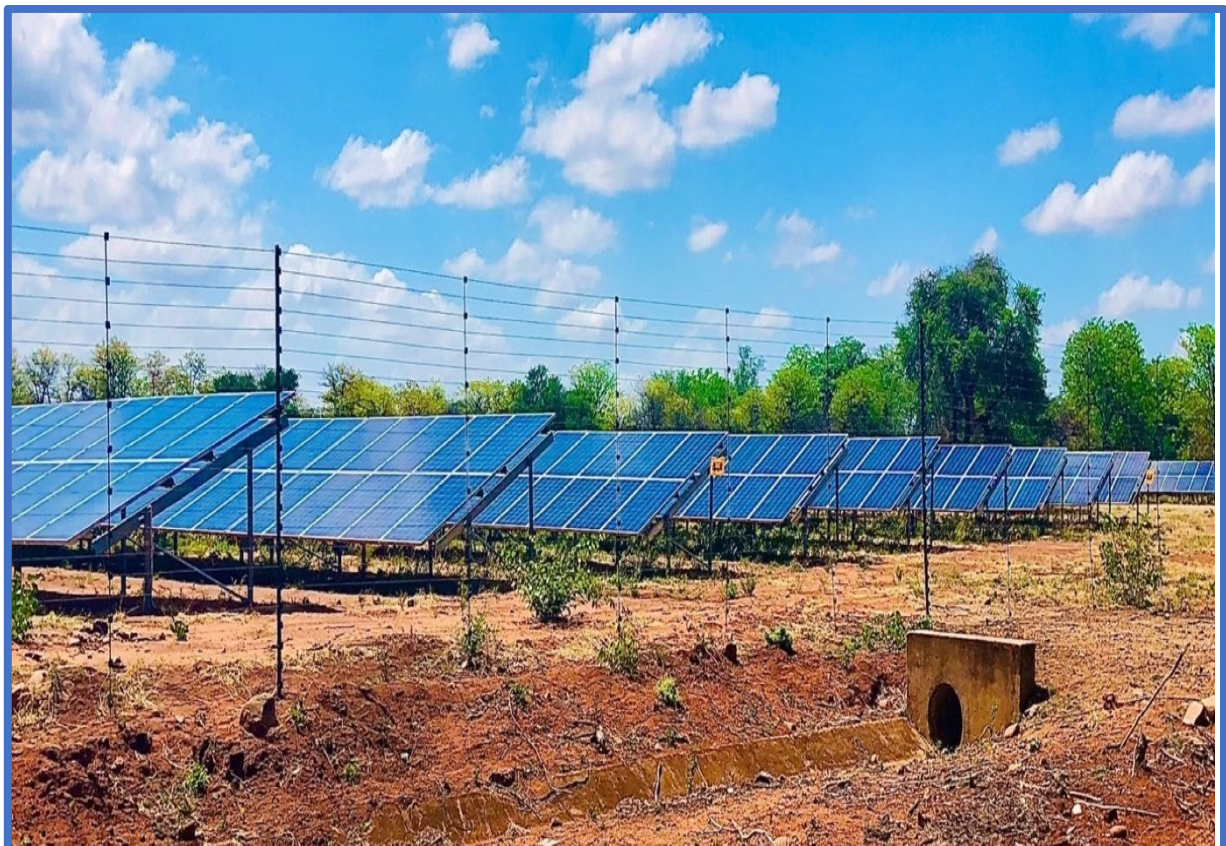
Figure 9 Photovoltaic solar panels (1 037 kWp) at TCM
