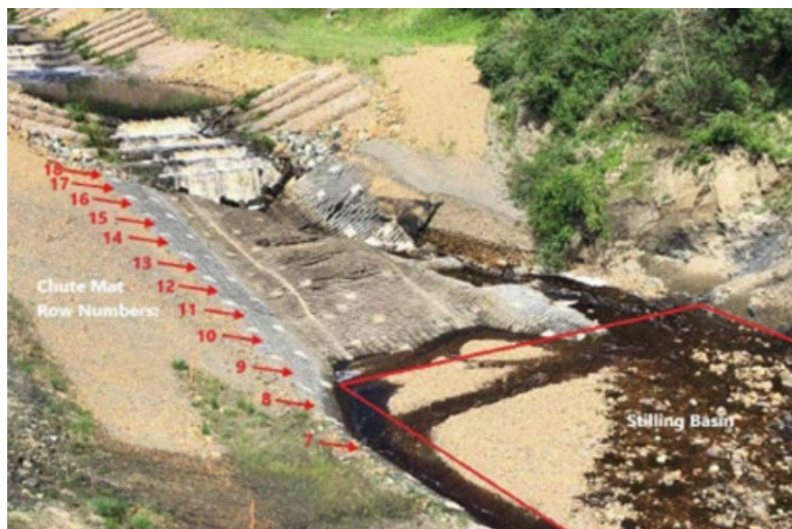
Figure 7 Failed configuration of the ACB mat chute structure in the spring/summer of 2018
