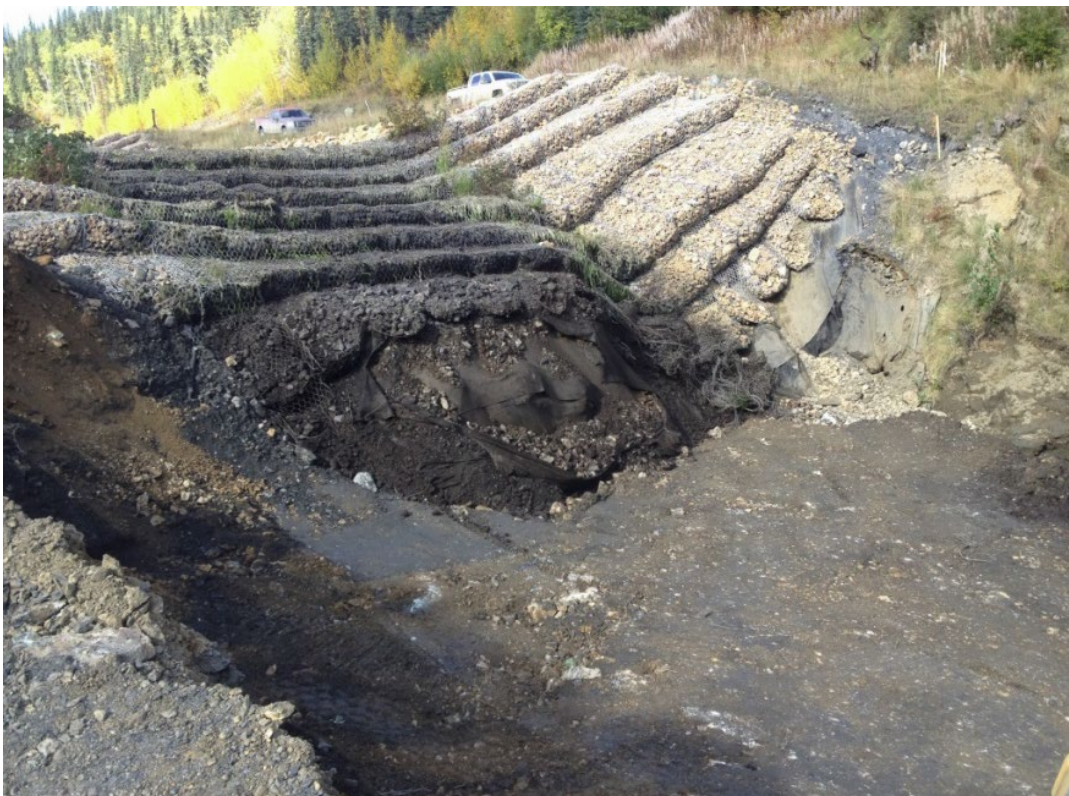
Figure 5 The failed surface of DS4 (ADVISIAN, 2015)
