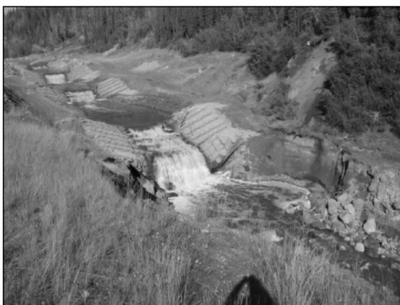
Figure 3 The failed drop structure 4 (DS4) following the August 2010 storm (Wingrove, 2011)
