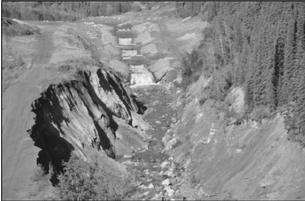
Figure 4 Additional failures in the waste rock slopes downstream of DS4 (Wingrove, 2011)
