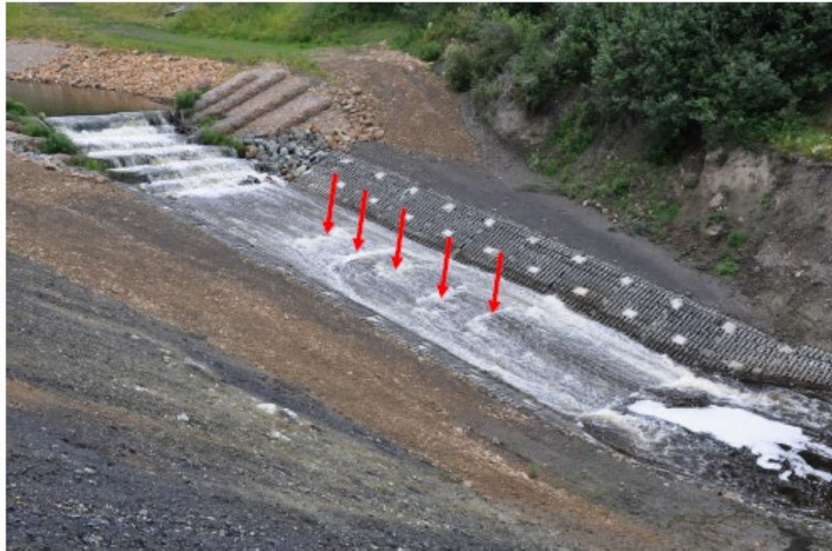
Figure 6 Displacements observed in the chute channel in 2016 (BGC, 2016)
