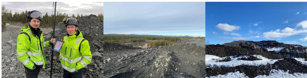
Figure 8 (a) Operators Håkan Jonsson (left) and Andre Stenman (right) planning the work ahead; (b) First ramp cut down to 360 on the existing waste dump; (c) Ongoing contouring and shaping of the test site using bulldozer
