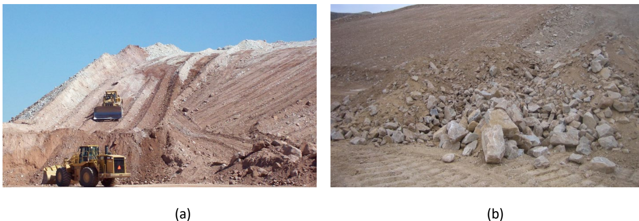
Figure 2 Reduction of rock content using mine equipment at (a) the dozer push and load-out area at the borrow stockpile with oversized rock in the lower right corner; (b) excessive rock removal/management at the toe of the slope during cover placement on slopes
