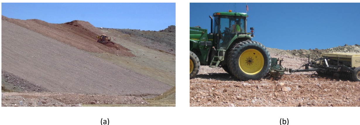
Figure 3 West Stockpile 3:1 sloped RLG test plot construction: (a) dozer placing cover materials dumped at the crest; (b) scarification of the cover using small rippers prior to drill seeding
