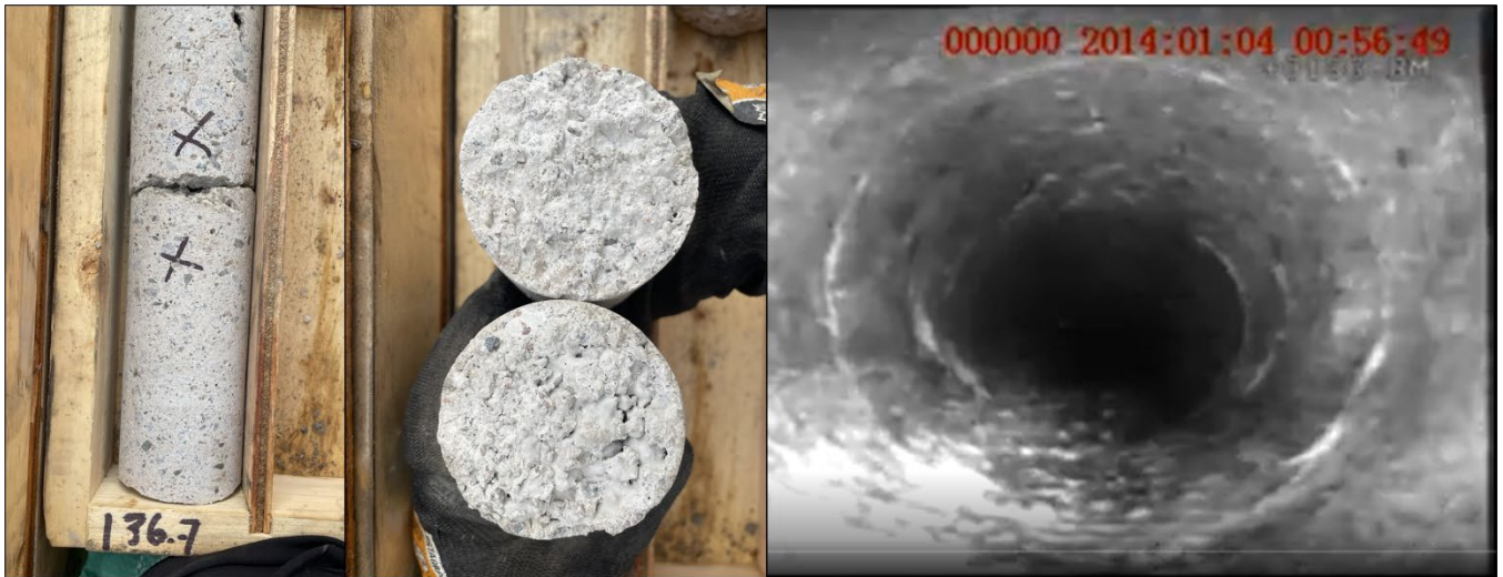
Figure 8 Interpretation cold joint in box (left), split to expose surfaces (centre) and in borehole camera video (right) from borehole 3 at 136.8 m along hole/ 27.18 mamsl
