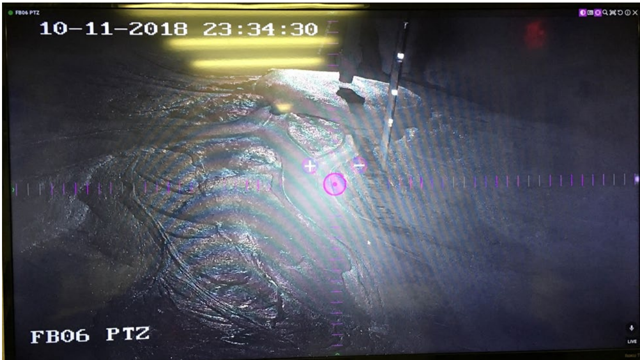
Figure 5 Footage from underground infrared camera showing splash pool under tremie pipe. Extensometer string with reflective tape shown in foreground of tremie pipe and braided flow channels in SCC
