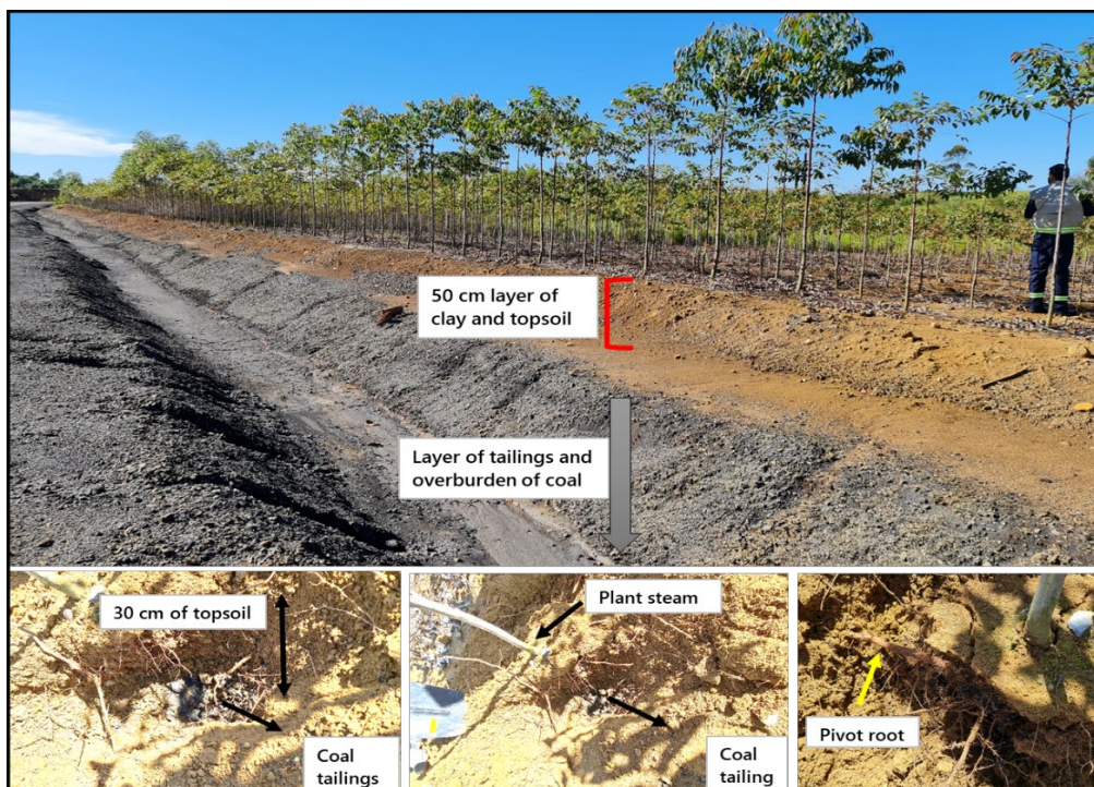
Figure 12 Rehabilitation of an area with coal tailings covered with 50 cm of clay and topsoil. In detail, the eucalyptus pivoting root coiling, avoiding contact with the tailings.
