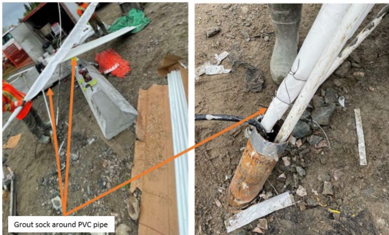
Figure 4 (left) Grout sock secured around PVC pipe prior to installation in the drillhole; (right) lowering the PVC pipe and grout sock into the drillhole for grouting
